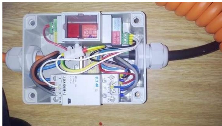
Picture 17: Charging cable made with EVSE DIN together with 4pole contactor in a box
